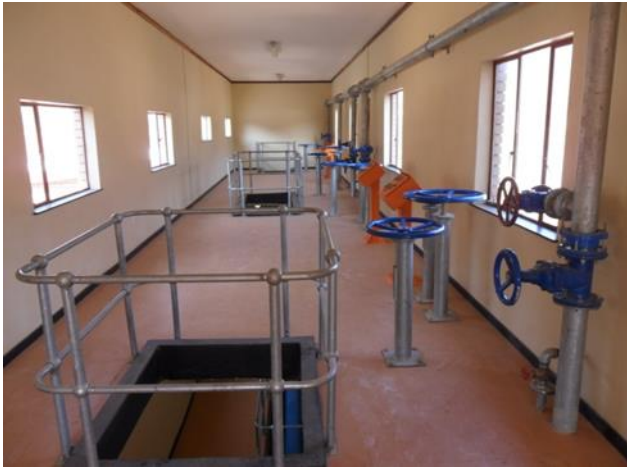
Pictures of Mutshedzi Water treatment plant
